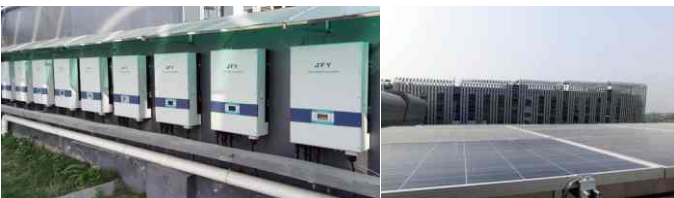
500kW On-grid PV Project in Shenzhen North Railway Station
