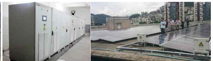
2.5MW Rooftop PV Grid Project in Guangzhou Industrial Park
