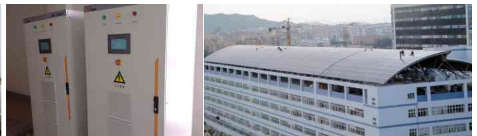
300kW Rooftop PV Project in Shenzhen Industrial Park
